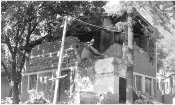
Figure 7.1 : A Damaged Building Due to an Earthquake
